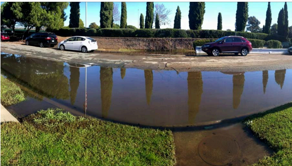
Figure 1.3 Veterans Court in the City of Alameda during King Tides. Groundwater intrusion into the sewer system provides a pathway for inland flooding when Bay tides are high. A high groundwater table and emergent groundwater flooding have caused pavement failures (May et al., 2023). (Photo credit: Kristina Hill)
