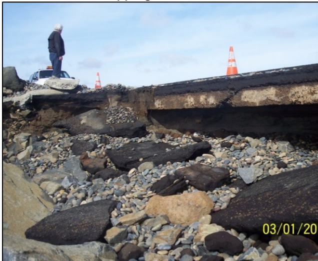
Wave-induced Damage to HWY 101
