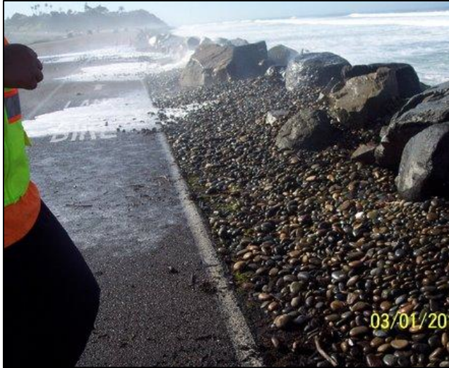
Overtopping of HWY 101
